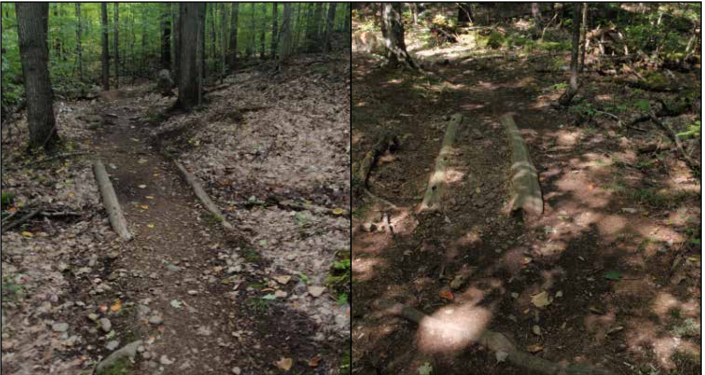
These pictures above show old style log and rock drainage structures built on The Flume mountain bike trail network in the Wilmington Wild Forest area.
