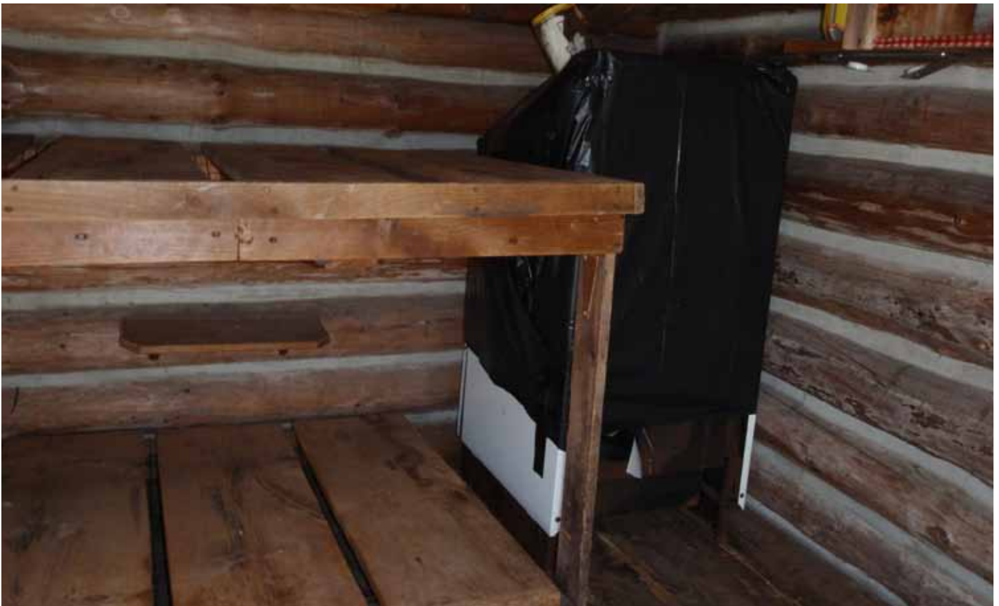
The Chub Pond Lean-to shows substantial modifications with shelves, bunk beds and various furniture strapped to the ceiling and stored in the lean-to. The lower picture shows a gas stove/oven stored in the lean-to.
