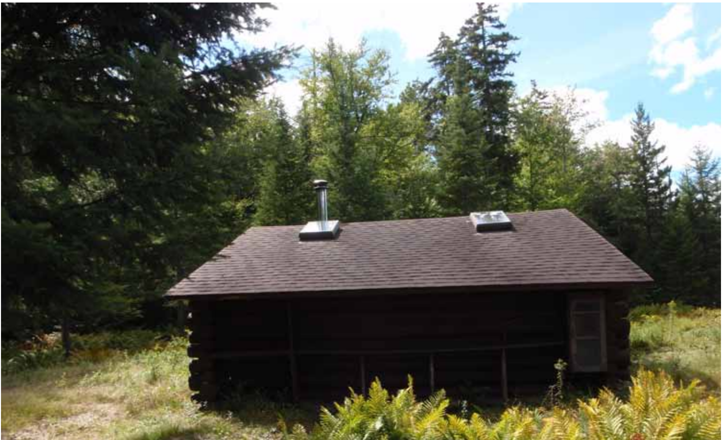
The top picture shows the Chub Pond Lean-to modified with a porch, railings and a chimney for a wood stove. The lower picture shows a new roof and skylights.
