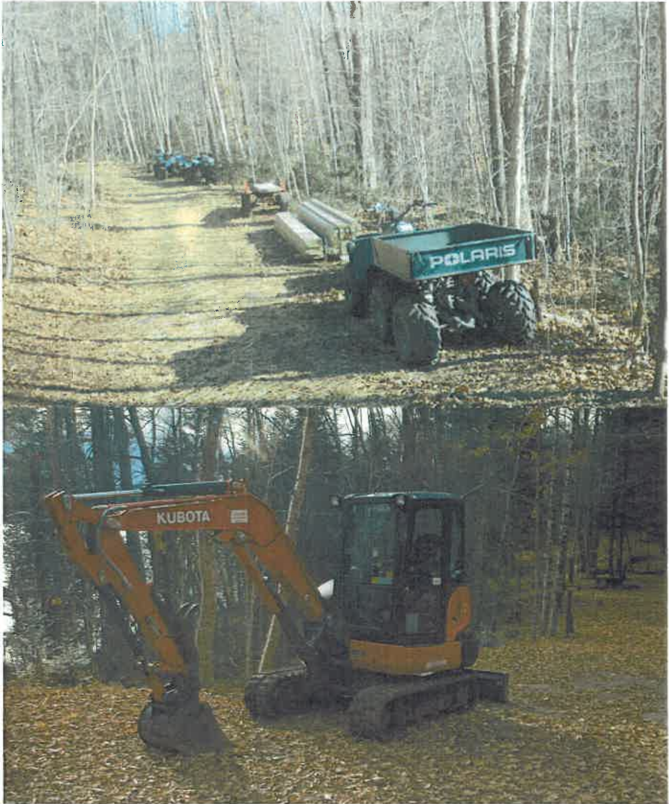
The pictures above show the heavy machinery used by the DEC to build new class II community connector snowmobile trails. Foot trails are built with hand tools.
