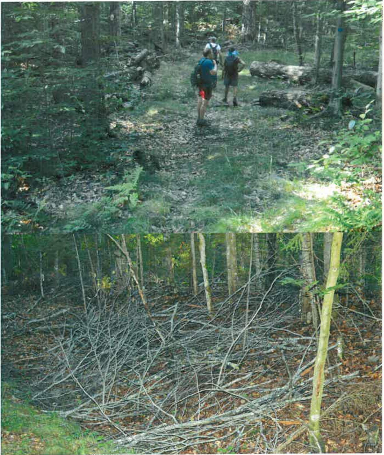
The pictures above were taken in the summer of 2016 on the Seventh Lake Mountain Trail, a newly constructed class II community connector snowmobile trail located in the Moose River Plains Wild Forest area, part of the Adirondack Forest Preserve. These pictures show trailside debris.
