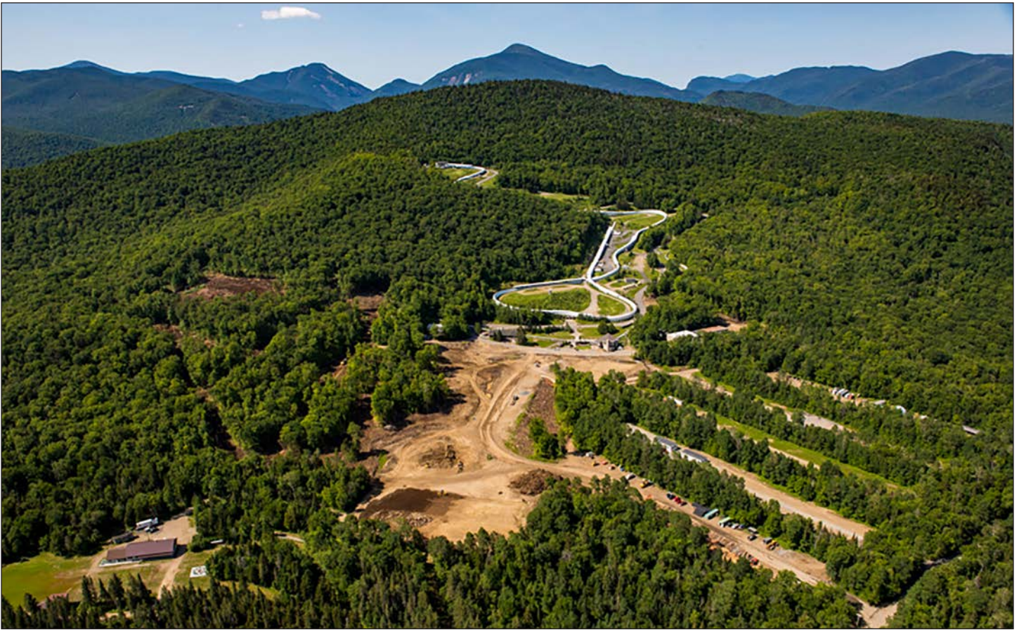
Parts of the Mt. Van Hoevenberg Winter Sports Complex under renovation. Construction activities are happening on both the Town of North Elba and Forest Preserve lands classified as Intensive Use and managed by the Olympic Regional Development Authority.
